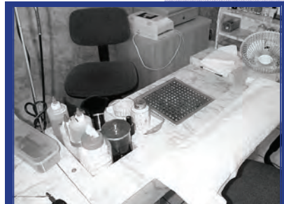
Exhaust vent embedded in nail care workstation
